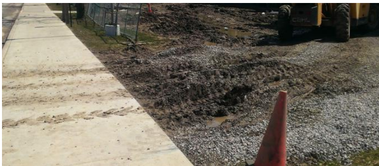
Improperly constructed construction entrance
